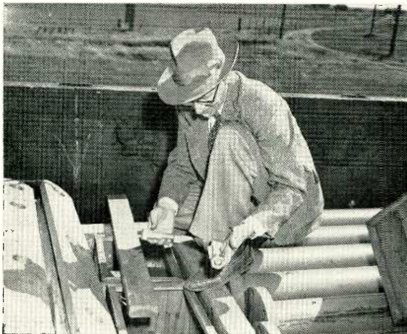
Engineer Ivar Nelson checks on parts of the supplies which are being used in the construction of the new KFYZ-tv antennae east of Bismarck.
