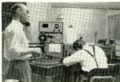
Control room—center of operations. Jim Schlecter (left) and Elmer Lee were on duty here during flood rush.
