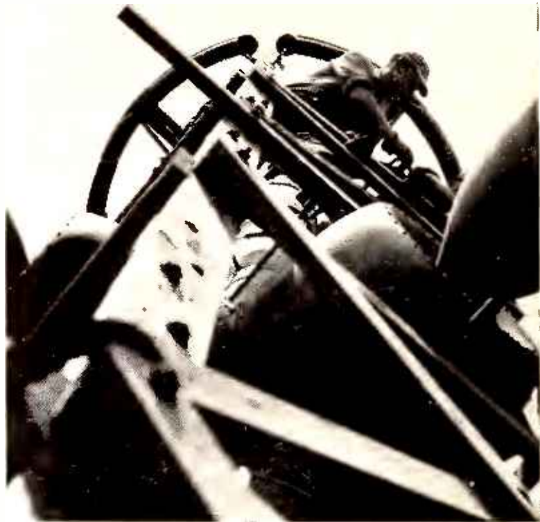
Steeplejacks at work on an NBC television antenna—1250 feet above the sidewalks of New York. Its height gives telecasts a wider range in the New York and New Jersey area.
