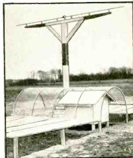
Above—The complete "signal" transmitter installed at the Indianapolis airport.
