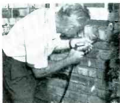
ABOVE: INVERTER-POWERED electric drill cutting hole into concrete wall to mount stud for leadin.
