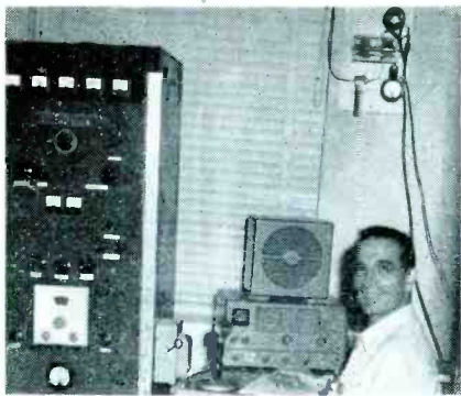
HAM EQUIPMENT installed and operated by Service Man Roulias, who is also a member of the Amateur Radio Emergency Corps for Public Service.
