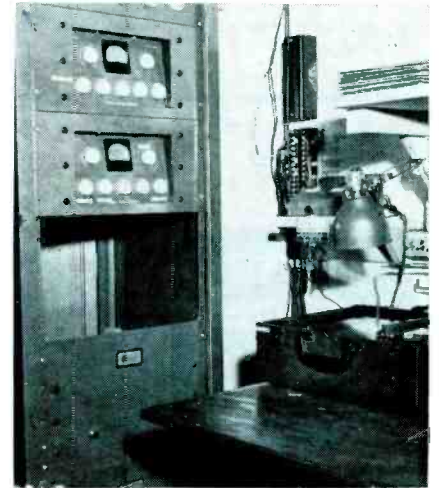
AMPLIFIER control panel and phono unit. Additional control equipment was added to rack after this photo was taken.
