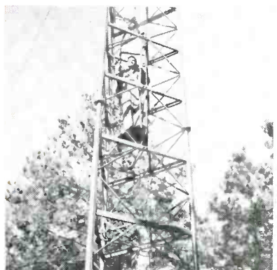
Triangular tower, designed for community TV, installed in Jacksonville, Texas. Tower features an elevator to facilitate inspection and maintenance of tower, and antennas and amplifiers. (Liberty Tower.)
