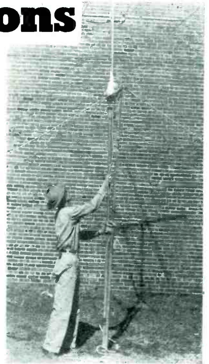
Mast and gin-pole just after erection. Mast and antenna are erect, being held by knot around both pole and mast. Guy wires, lead-in and rotator cables, omitted in this illustration for pictorial clarity, should be attached while mast is still resting on shears, before raising.
