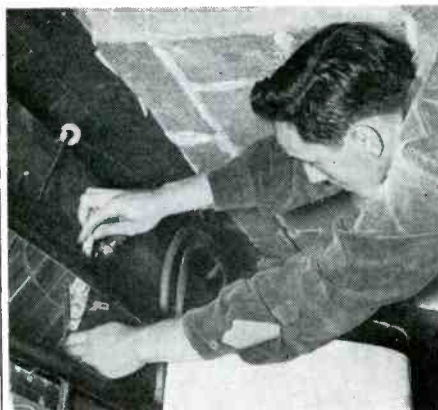
Fig. 6. Installing a lightning arrester on the cold water pipe in the basement.
