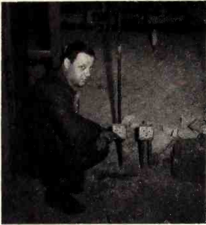
Fig. 3. The amplifier cabinet will finally be flush with the wall which will be built after all the conduit is in place.
