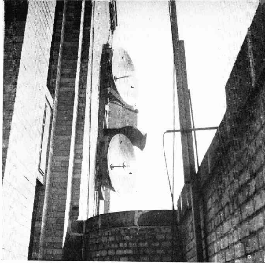
Receiving and transmitting 1200 mc Multi-channel link antenna installation atop the International Telephone and Telegraph Corporation building, New York City, for the Pulse Time Modulation System developed by the Corporation's associate, Federal Telephone and Radio Corporation
