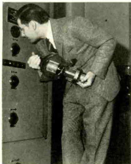
Ken Gardner, Chief Engineer of WHAM-W51R, checks up on the final amplifier in Rochester's 3-kw FM job, W51R. The circular peep-hole allows a safe look at the cherry-red plates of the 1500 Ts
