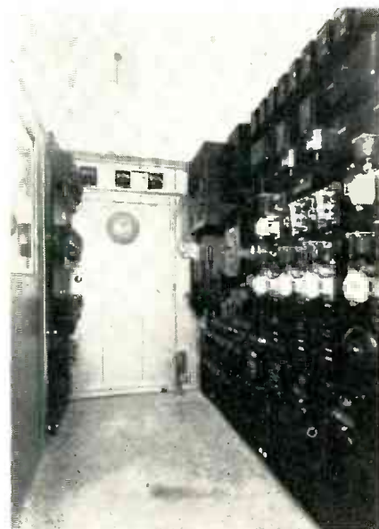
All power switches and control and overload relays of the transmitter are centrally located in this compartment. Situated behind the middle door of the transmitter enclosure, the control compartment can be entered during operation of the equipment for check-ups on the control circuits.
