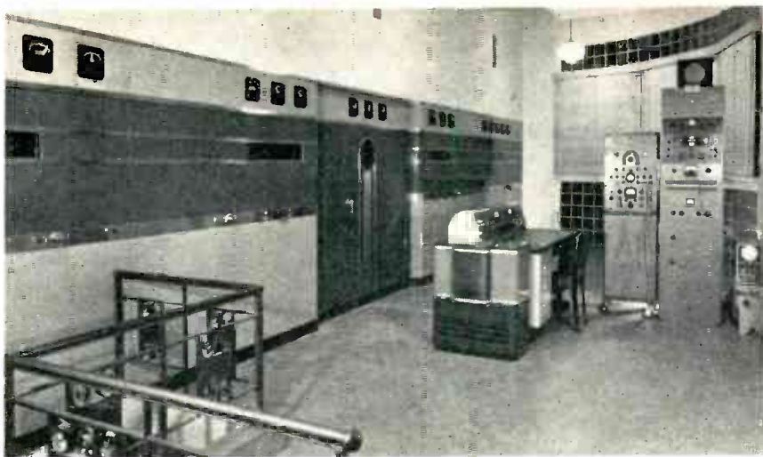
This view inside the building shows the front of the RCA 50-kilowatt international shortwave transmitter, with the console table, monitoring and measuring equipment, limiting amplifier, hum buck amplifier, and speech input equipment for emergency operations. Center door of transmitter enclosure leads to control compartment, inner doors on either side give access to the two radio-frequency channels, and the outer doors lead to the fronts of the exciter units.
