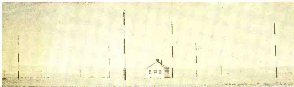
MRL antenna installation. The range transmitter is located in the building at the center of the four loop-type antennas.
