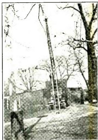
2 Six helpers; six ideas as to how it should be put up.
