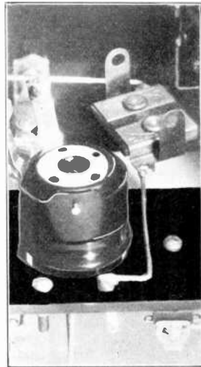
A VERY POOR WAY TO MOUNT A GRID CONDENSER
