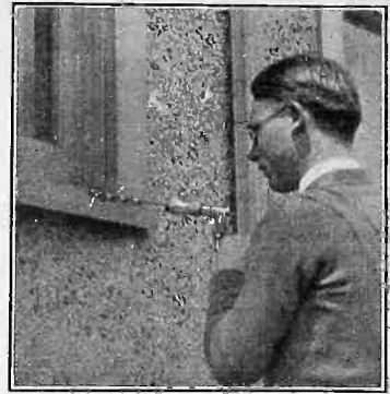
DRILL a hole for a lead-in insulator tube so that the hole slants upward from the outside. When it rains the water will not drop into the house.
