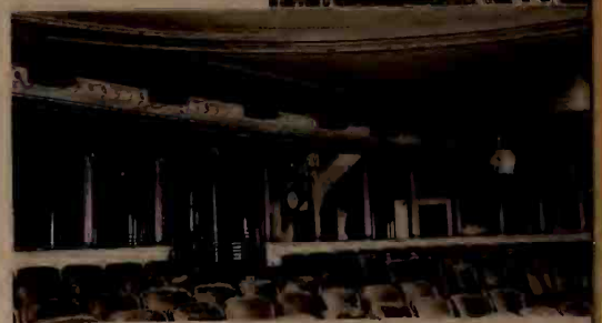
Top. One of the "house" speakers being installed in Broadway Theatre, New York.
