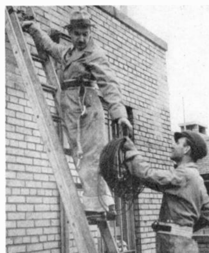
★ Servicemen installing a master antenna system atop an apartment building. Note that they wear safety belts—a worthwhile precaution when working on tall buildings. See article on page 4. (Photo by Austin C. Les-carboursa)
