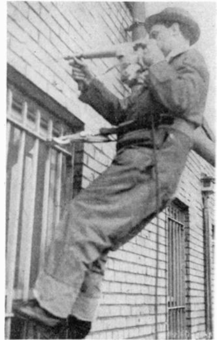
Serviceman working with small electric jack hammer, boring holes in masonry. Note safety belt.
