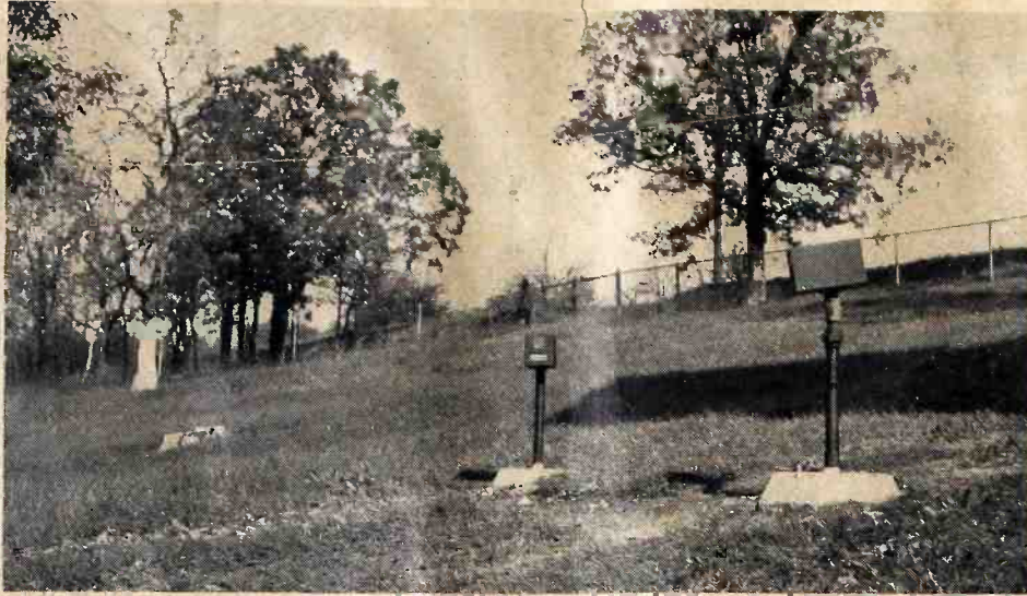
TYPICAL WORNER PHOTOELECTRIC ANTI-SABOTAGE INSTALLATION.
