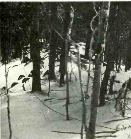
Coaxial cable which brings the signal down the hill from the remote-antenna site can be laid on the ground, as shown here.
