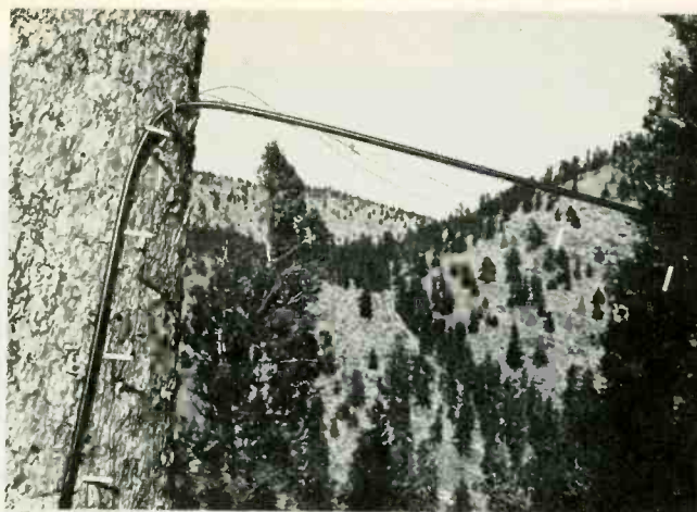
Coaxial cable replaces ladder line, which required frequent repairs and, consequently, caused TV-reception outages.
