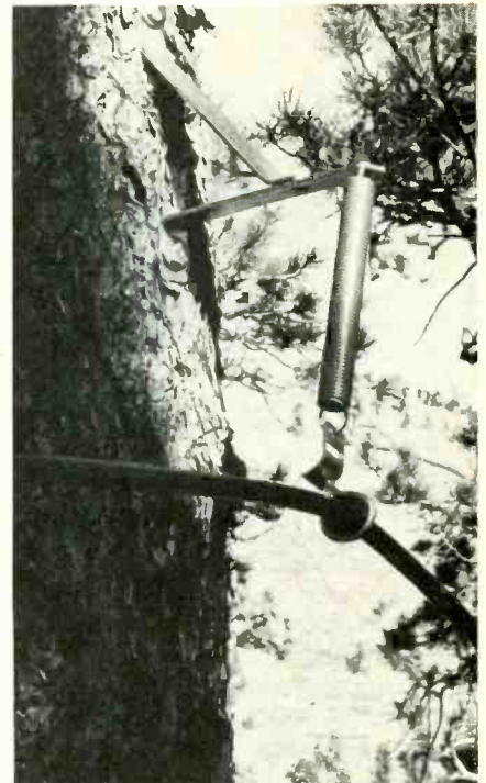
Coaxial cable may be strung between trees in wooded areas where foot or vehicular traffic might cause damage if it is laid on the ground.
