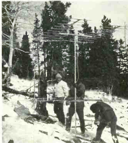
Technicians, working at 10,000 feet, ready a WS-1010 antenna for mounting on the lower mast section (next to stump.)
