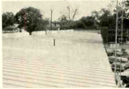
This vast expanse of roof is completely protected by pressure switches underneath.
