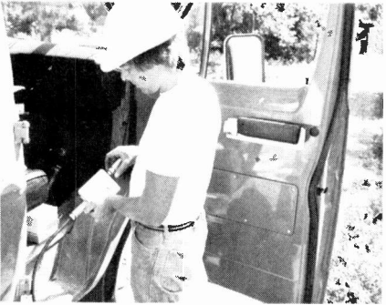
Fig. 3—Gast, owner/operator of Mike's Antenna Service, is shown here connecting a multi-tap to one of the .412 underground trunk cables he is installing in the mobile home park. All cable in the park is run underground.
