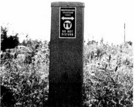
Fig. 4—Pedestal type enclosure which houses one of the multi-taps Gast is using to split and tap off the signals from the underground trunk cable.
