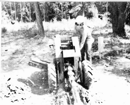
Fig. 5—Pete Wunsch, an employee of Mike's Antenna Service, is shown cutting a trench for the underground cable. Note multi-tap pedestal behind Wunsch.
