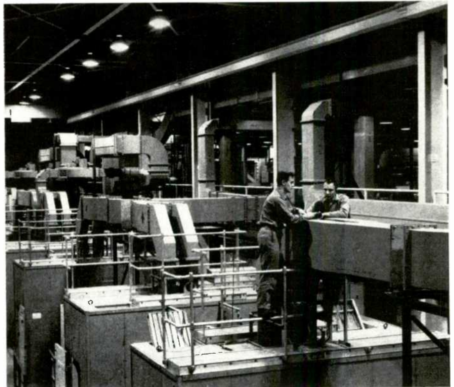
Fig. 3—GE technicians, Robert Morse, left, and Elnor Schilling, right, inspect waveguide sections which will carry r-f energy from transmitter power amplifier cabinets to scanner building. Nine-foot high klystron tubes are used in power amplifier.
