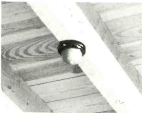
Fire sensor installed on rafter in Heisler's Dairy Bar Warehouse.
