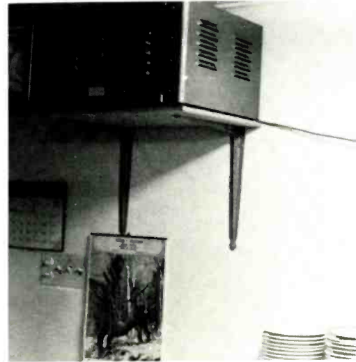
Control unit mounted on a shelf in the White Diner kitchen.
