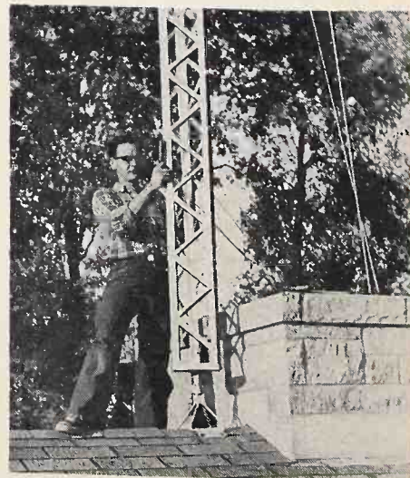
Fig. 4: Helpers adjust guy wires as tower is plumbed with a hand level.
