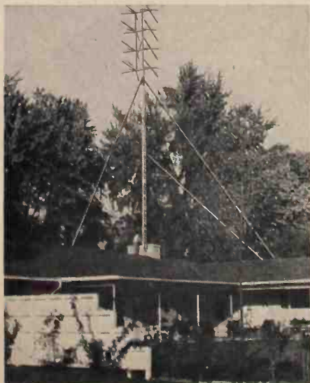
Fig. 5: The complete installation. A separate conductor should be run to a good ground for lightning protection. Grounding a guy wire endangers the mast, should that guy wire be damaged by lightning.
