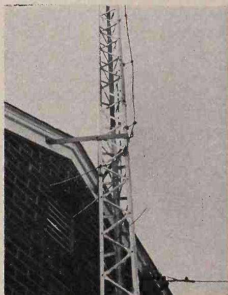
Fig. 2: When towers of up to 30 feet in height are installed next to a building, a single bracket attached to the gable or wall at a height of fifteen feet or more will take the place of all guy wires.
