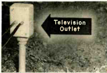
An outdoor tap in a buried-cable system, often used in motel jobs.
