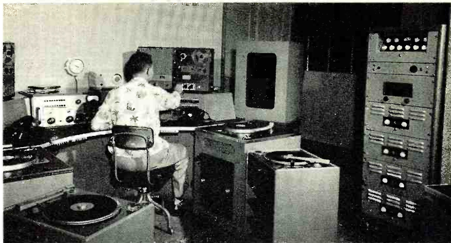
The "heart" of the Fair's elaborate sound system is located in Building 7A. The amplifiers, turntables, tape recording equipment, "beeped" FM receiver, preamps, mixers, etc. are of the latest design to provide coverage of the 500-acre site.
