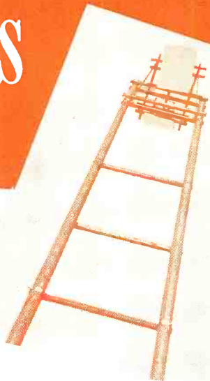
Top section of "H" fixture microwave antenna-supporting structure. 100 ft. wood poles are used. Plane reflectors, 4 by 6 feet, are mounted on top and reflect microwave beam from 4 ft. parabolic antennas below. This is part of the Rock Island's microwave communications system from Norton to Goodland.
