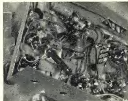
Under-chassis view of the r.f. section of the unit. Power supply is on other end.
