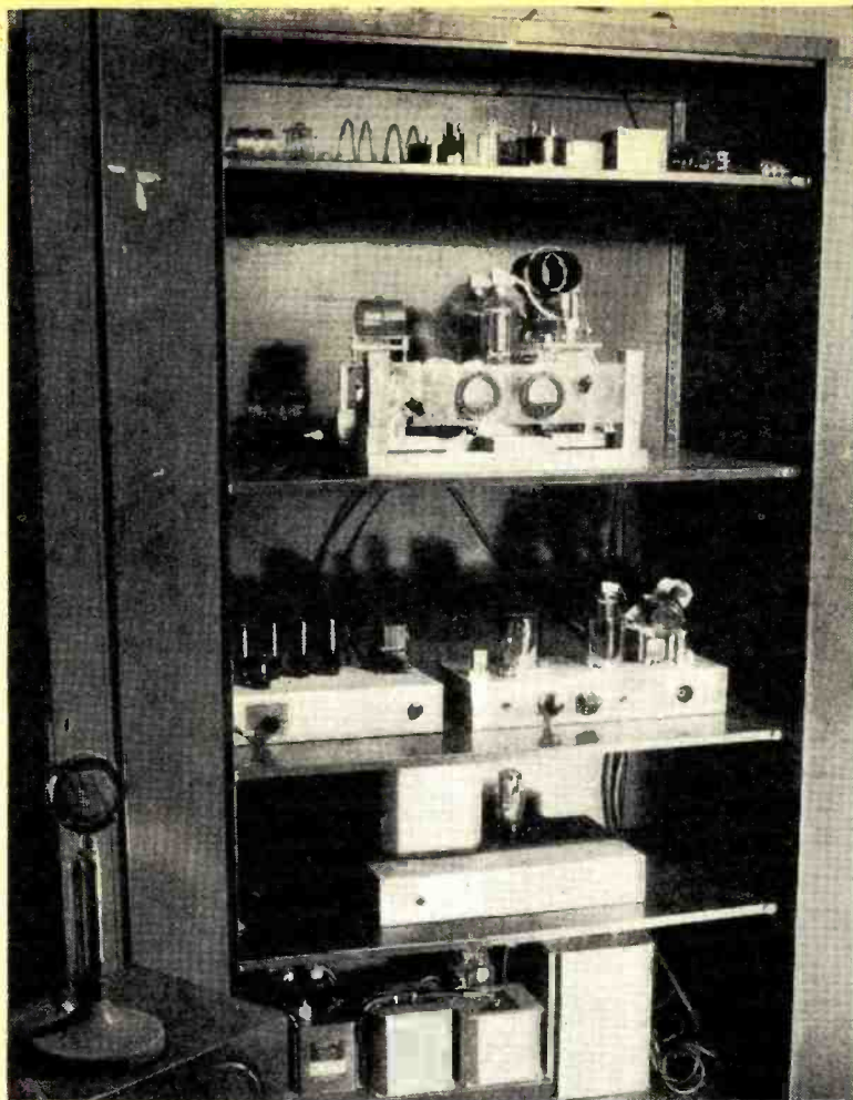
Fig. 1. Front view of transmitter. Compare with layout sketch of Fig. 4 for identification of the various stages. Safety grille has been removed from bottom shelf to show the high-voltage power supply.
