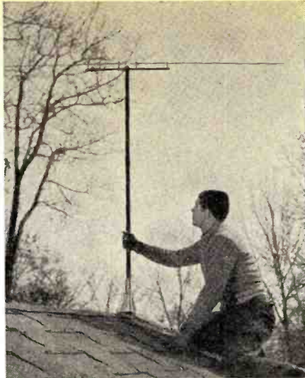
Fig. 8. Dipole assembly mounted permanently and roof installation completed. Fastening lead-in in place is next step.
