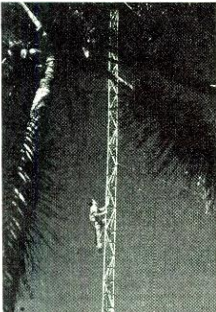
An AACS maintenance man goes up an antenna at one of the Gypsy Task Force Bases.
