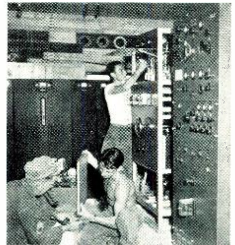
Three radio installation technicians put the finishing touches on 10 kw. transmitters at AACCS master station, Miami.
