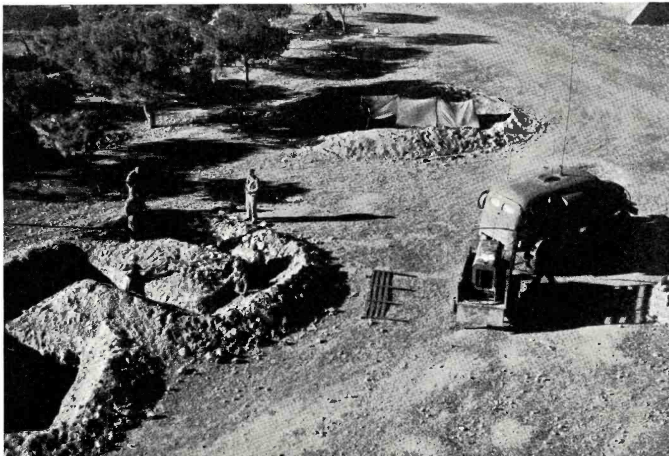
Members of U. S. Aviation Engineers building shelters near air field in Youks Les Bains, North Africa. SCR-299 on right.
