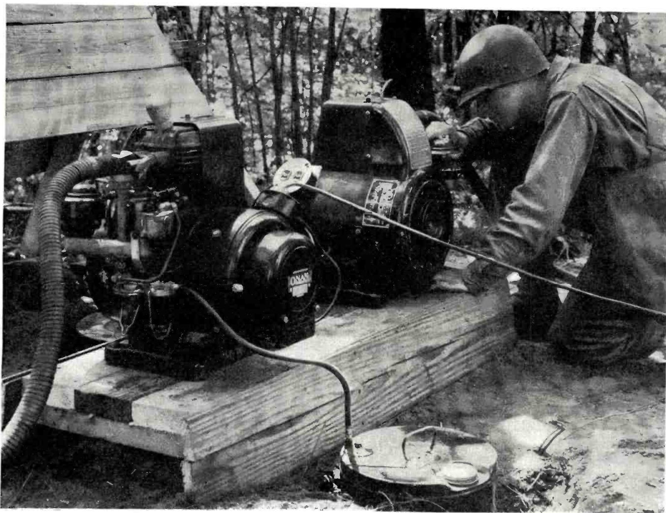
Five-hundred watt power unit supplying 110-volts a.c. for electric lighting and communications equipment.
