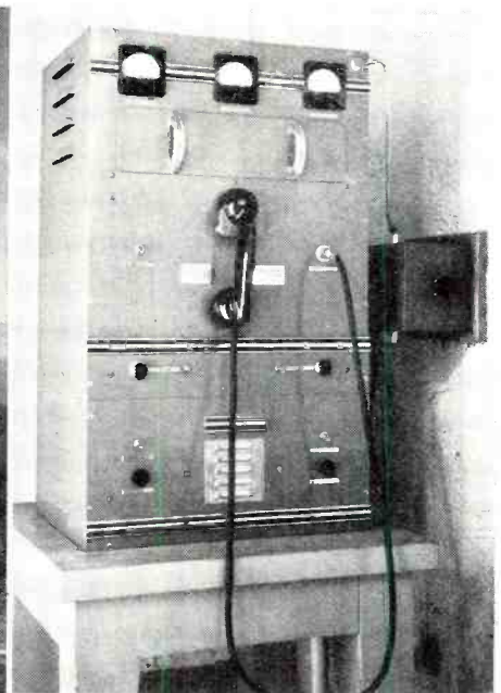
100 watt radiophone transmitter at the fixed station nerve center.
