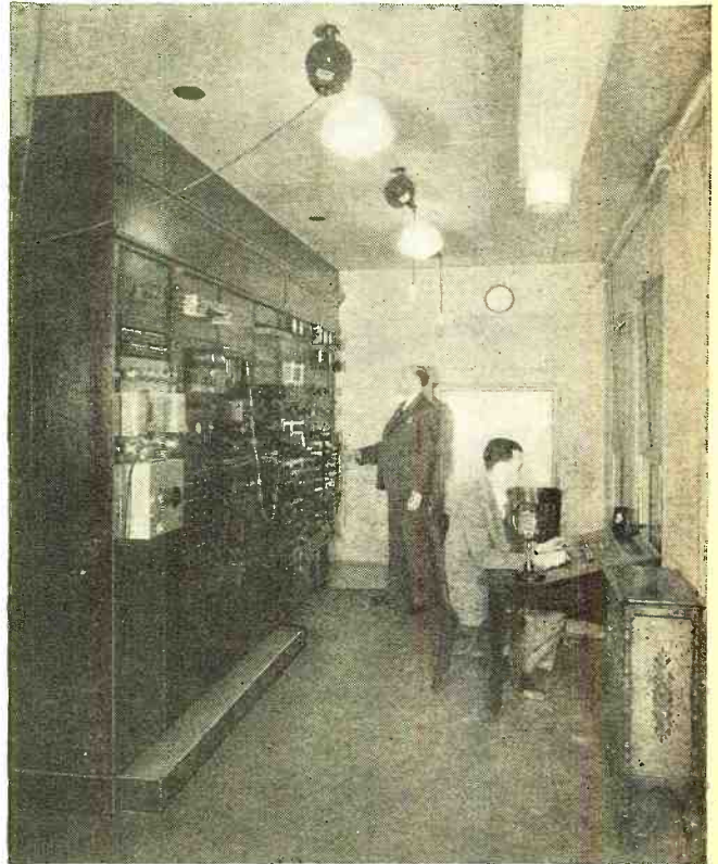
The control equipment of a modern station, showing the complicated panels and switches. The scene is in the control room of the Times Square studios of the National Broadcasting Co. At the switchboard is W. S. T. Redfern and at the monitor table Richard Stoddart
