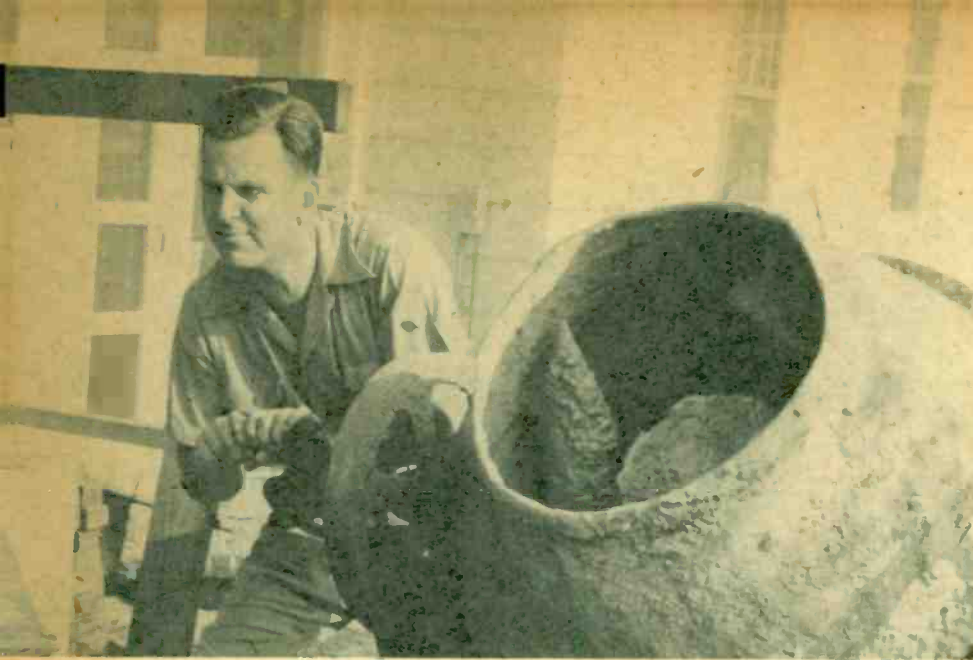
LEWIS CHOSE A FARM site on the banks of Patuxent River in the heart of historic St. Mary's County, Maryland. Here he's lending a hand at cement mixing.
