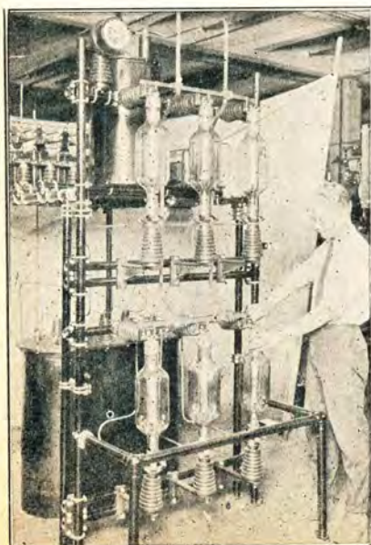
KENETRON RECTIFIER UNIT FOR THE 20 KW SET.
