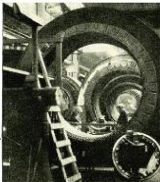
Uniform durable insulation is vital to the satisfactory performance of the stationary armature for this G-E 30,000-kw. synchronous condenser
