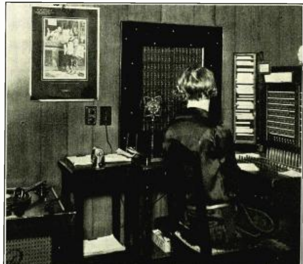
Showing telephone and selective call switchboard in Hotel Hoffman, South Bend, Indiana.
