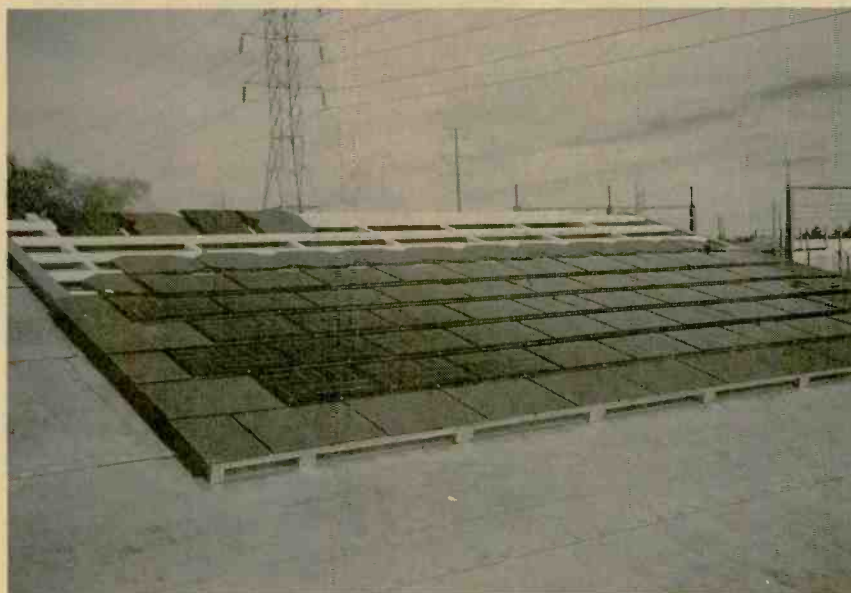
Part of a SunSlate-roofing-tile power array installed at the Arizona Public Service Company's STAR Center in Tempe, AZ. The complete system is rated at one kilowatt.
