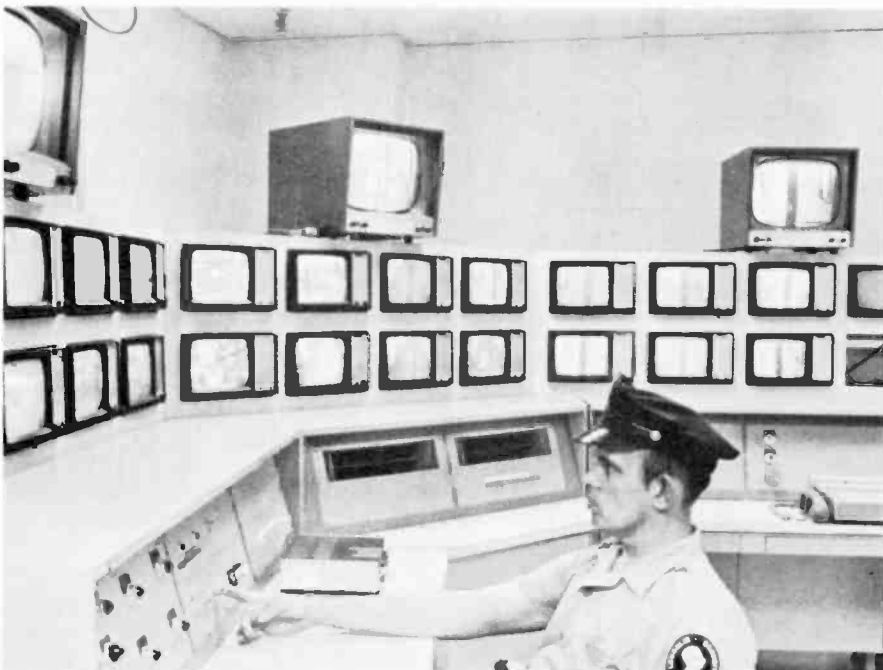
BANK'S SECURITY GUARD monitors some of the 30 CCTV cameras in First Maryland Bank building. This frees other guards for more vital roles in bank's security system.
