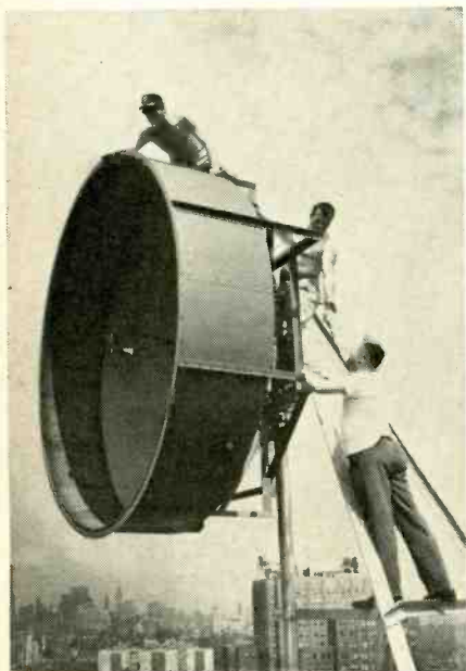
Workmen erect a microwave antenna on Western Union's 24-story headquarters building in New York.
