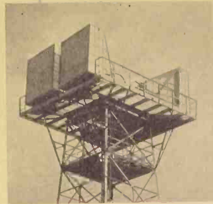
A typical lens antenna system shown mounted at the top of a steel tower.
