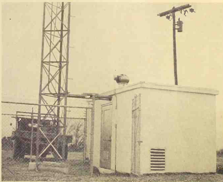
One of the microwave relay stations of the Texas Eastern Transmission Corporation.
