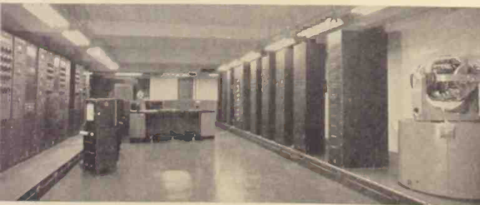
Part of Project Cyclone, one of the world's largest analogue computer installations, designed and built by engineers of the Reeves Instrument Corp.
