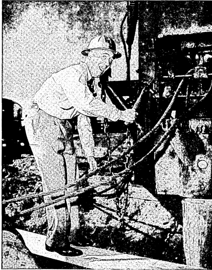
Gayle V. Grubb, manager of KGO, San Francisco, gave a 50,000-watt wallop to the pile driver's job of 'planting' the first piling for the station's new high powered transmitter. Scheduled to go on the air January 1, the new KGO transmitter will cost an estimated $400,000.
