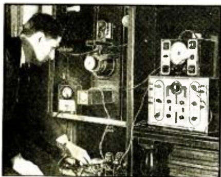
Fig. B. The rear view of the equipment.
