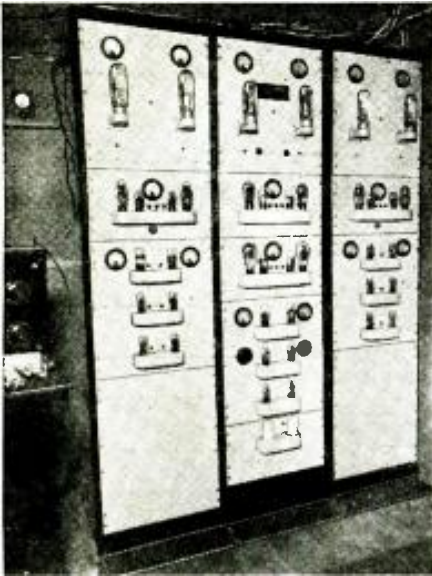
Fig. G Two amplifiers are mounted on three racks.
