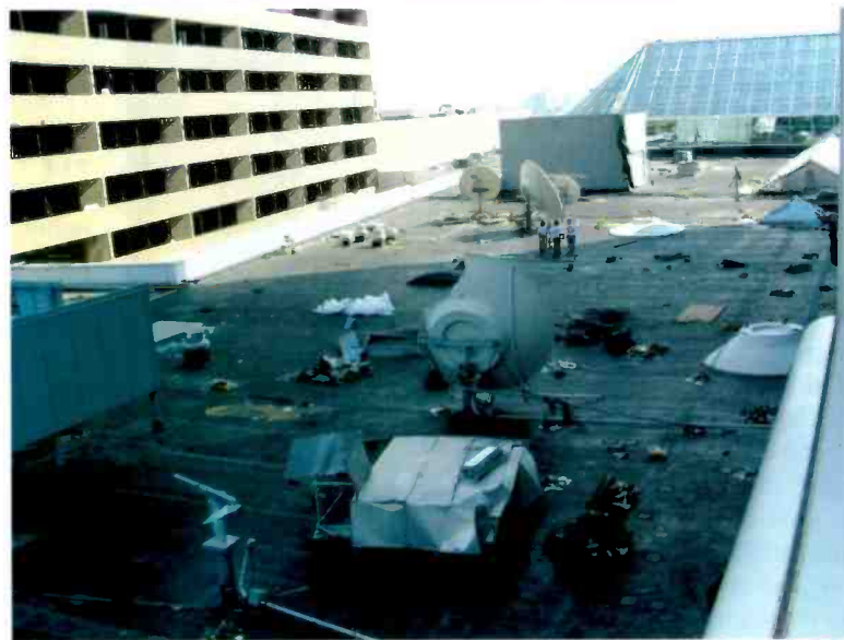
One of the many damaged offices at Entercom's cluster in the Dominion Tower, as well as Entercom's damaged satellite gear.
