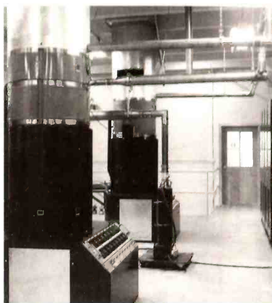
The final amplifiers with eight tubes each—part of the WBCT-FM RCA 500kw ERP transmission system, circa late 50s-early 60s.
