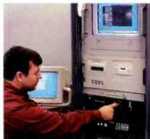
USADR's on-site IBOC transmission system
