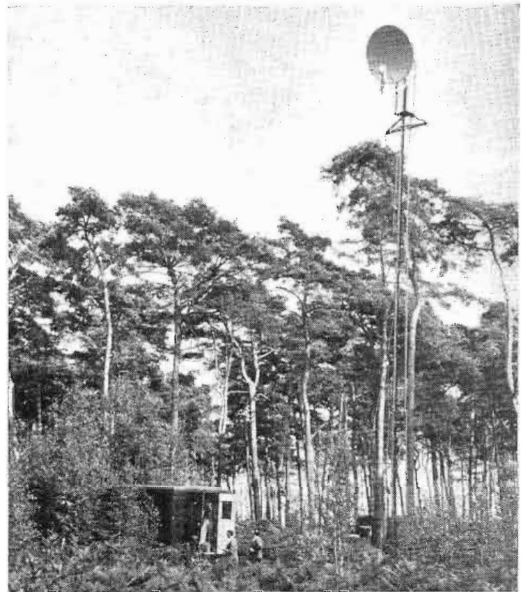
This microwave antenna, located at a secluded operations base in Western Europe, is one of the links in an RCA radio network linking Allied air installations with Central Europe headquarters of the U. S. Air Force.
